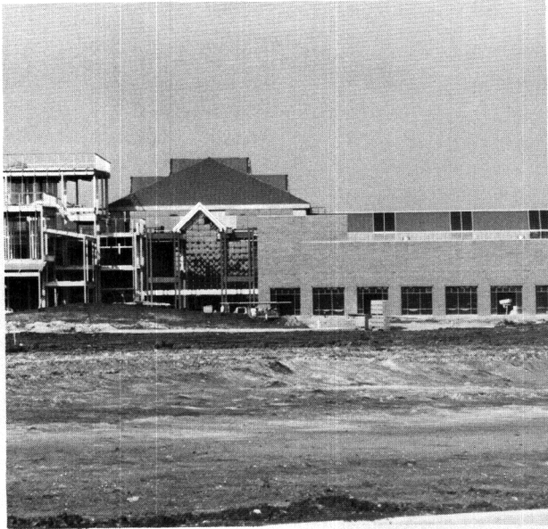
The east end of the building was almost completely bricked in by January 1988, with work progressing on the theatre (left).
