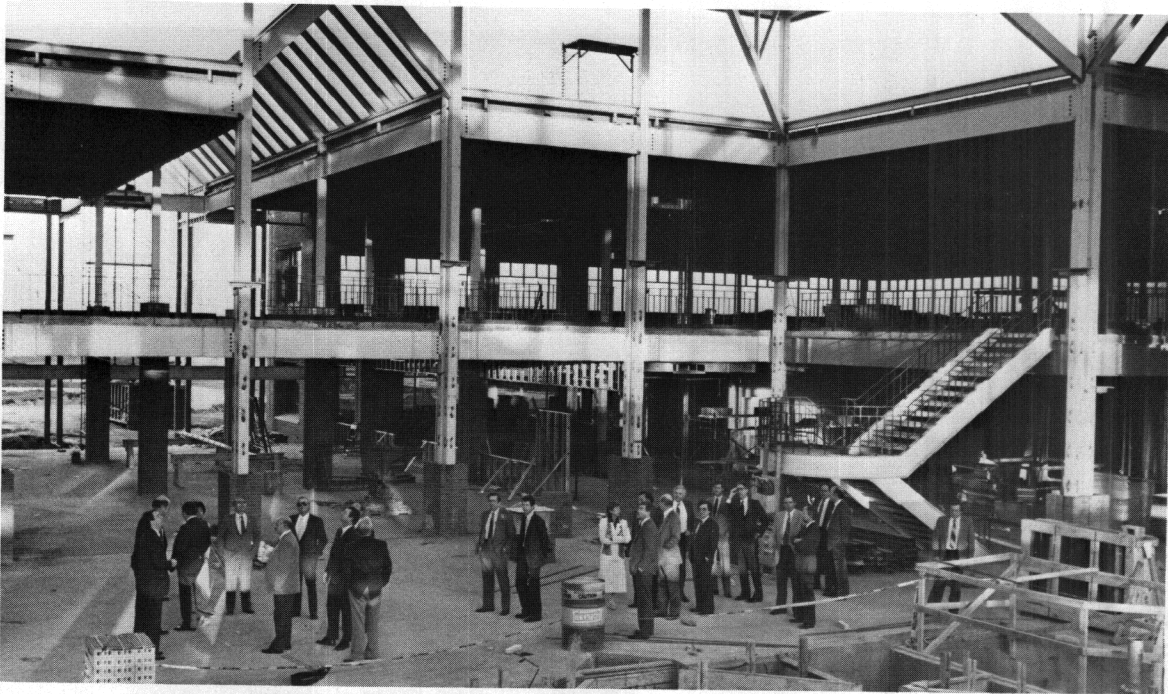
Civic leaders and CCCC Board members toured the campus in February, 1988. Pictured is the main courtyard, with fountain construction in the foreground.
